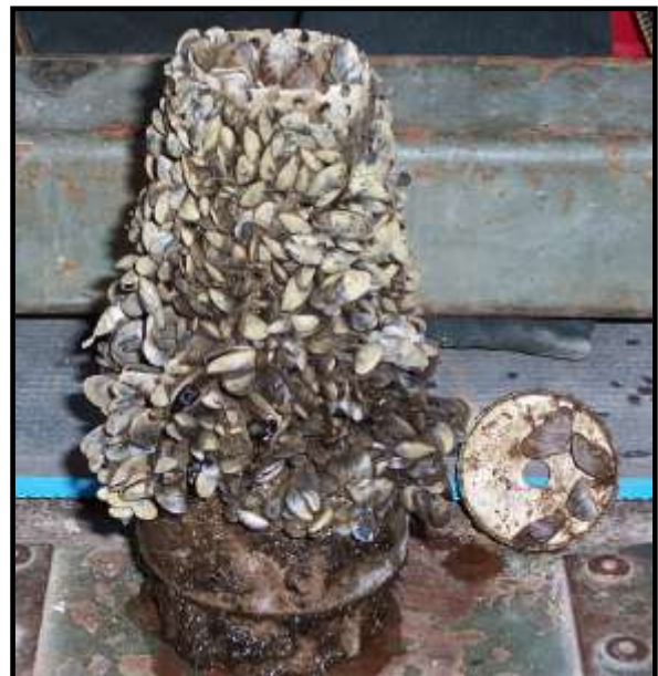
Figure 6 – Zebra Mussels can clog a water intake (foot valve) if you don’t clean it off regularly
